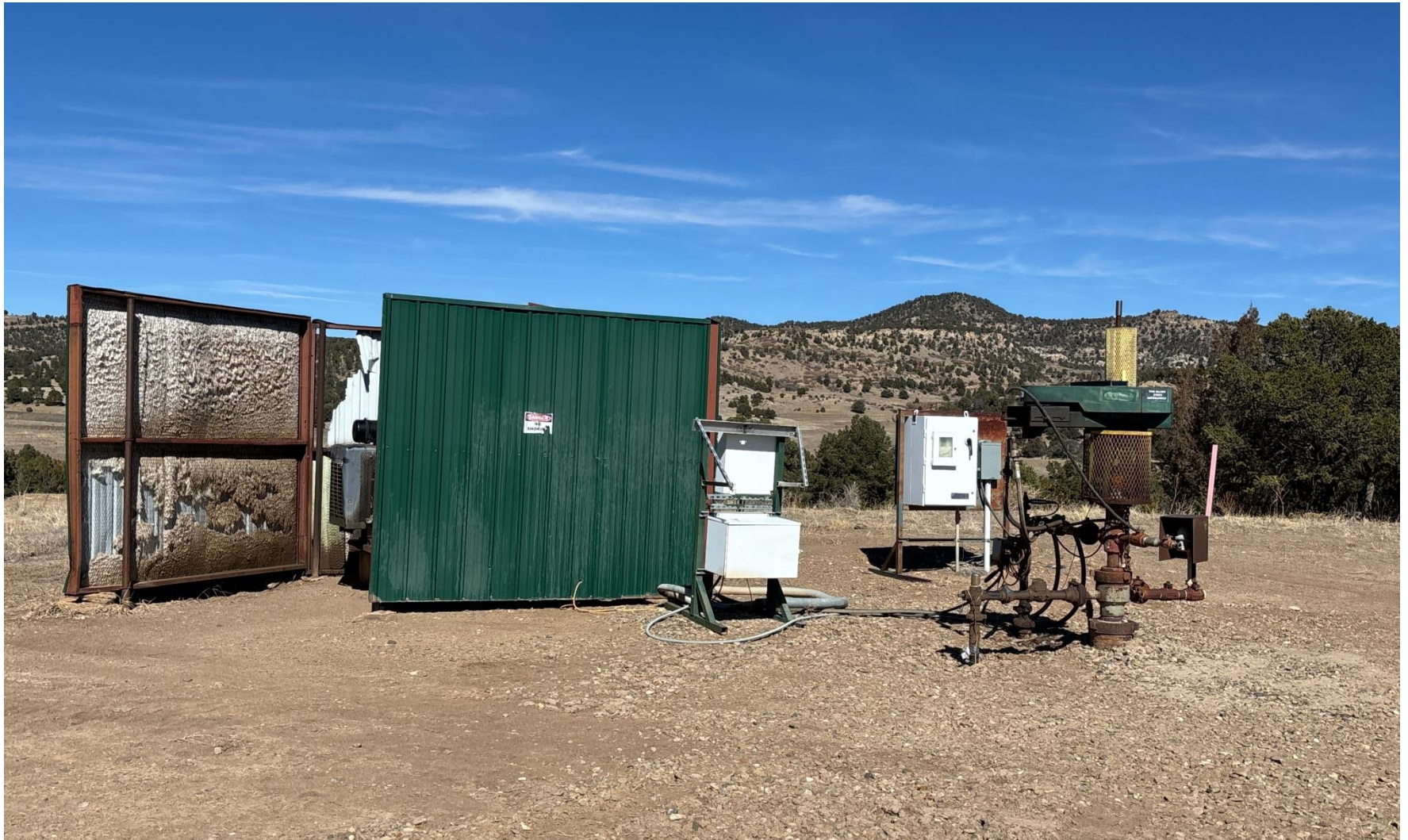
PHOTO 3: WELLHEAD AND EQUIPMENT.
