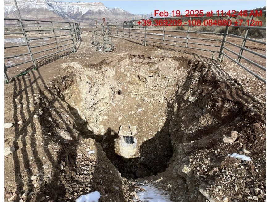
Photo # 5333 Open hole with no wildlife egress/wildlife hazard
