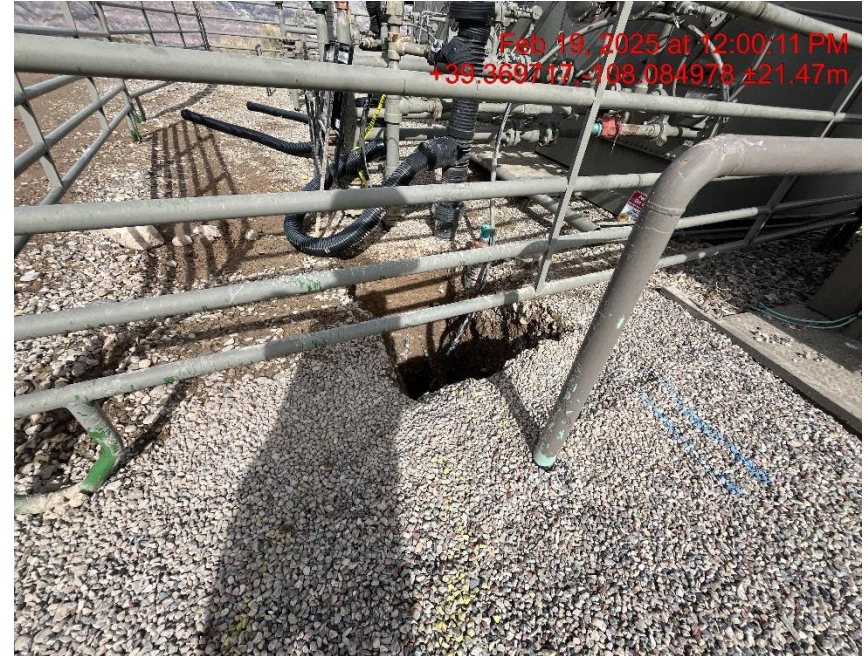
Photo # 5345 Open hole with no wildlife egress/wildlife hazard
