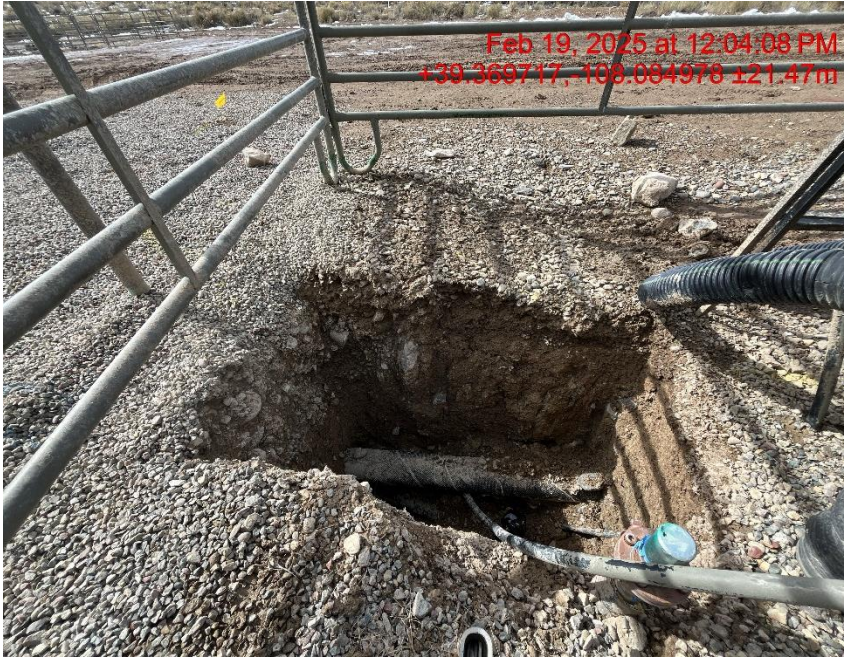
Photo # 5349 Open hole with no wildlife egress/wildlife hazard
