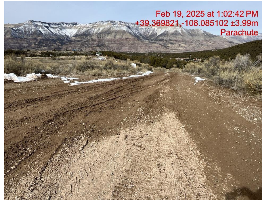
Photo # 5417 Tracking onto lease road/Insufficient tracking BMP's
