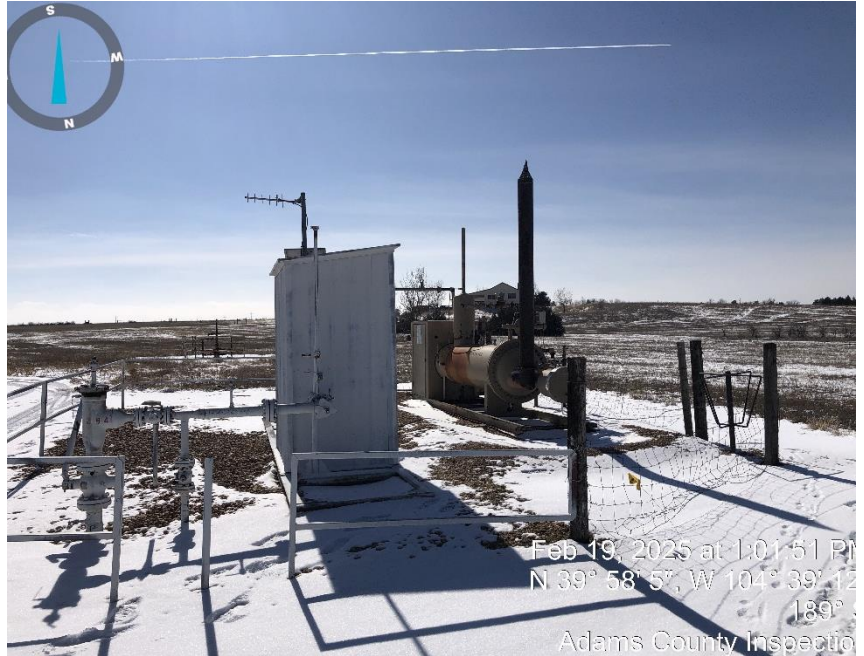
Photo#2 Meter house & Separator.
