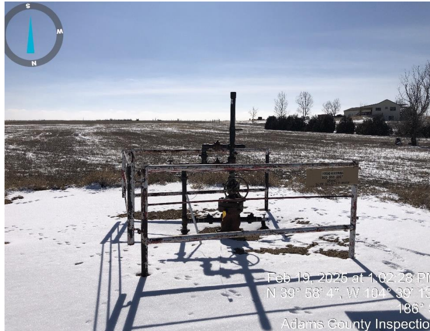
Photo #3 Well head.
