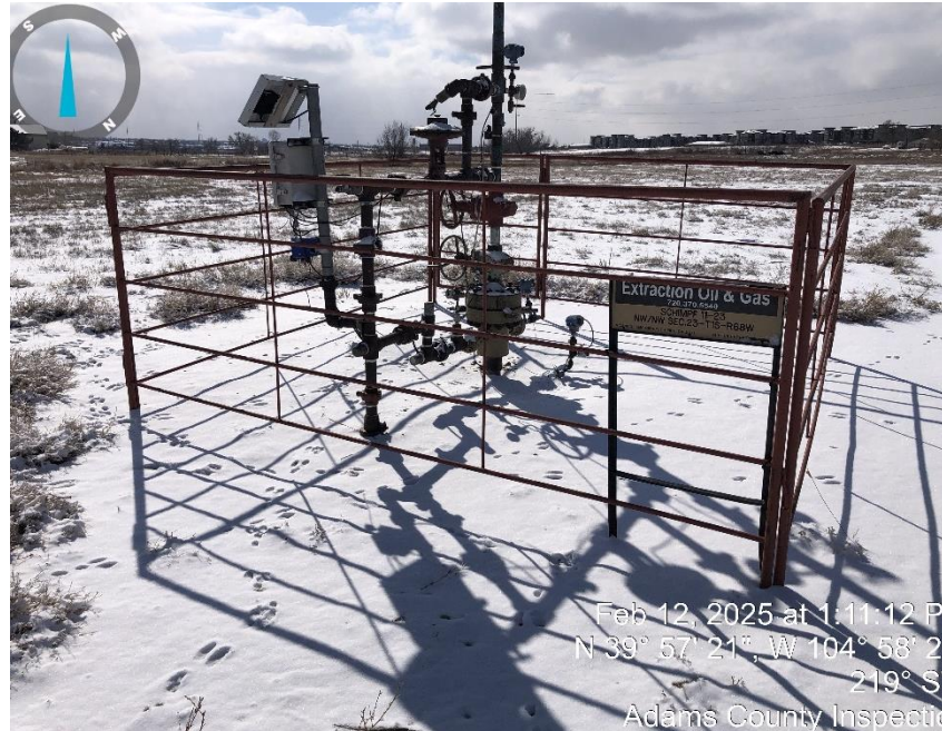
Photo #3 Well head.
