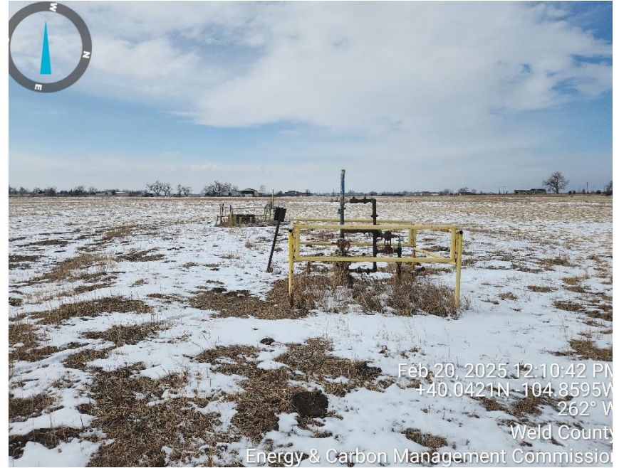
Photo 2 well head and equipment
