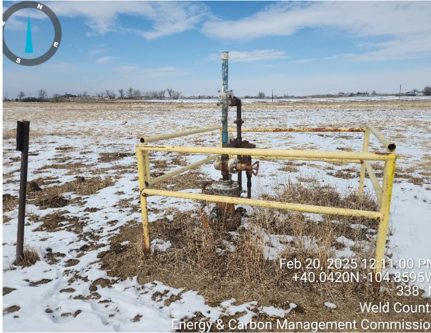
Photo 1 well head and equipment
