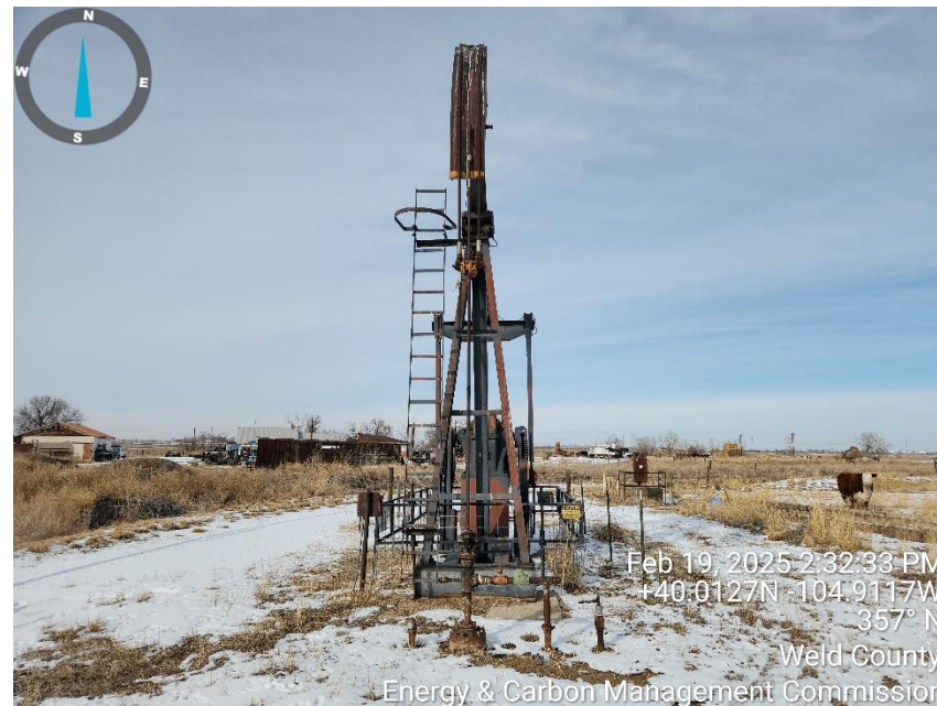
Photo 2 well head and equipment
