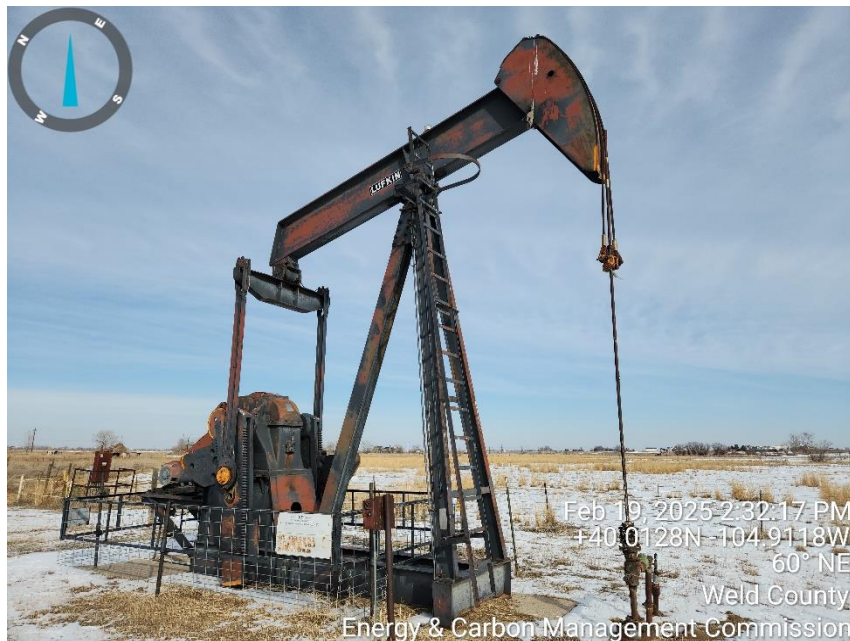
Photo 1 well head and equipment
