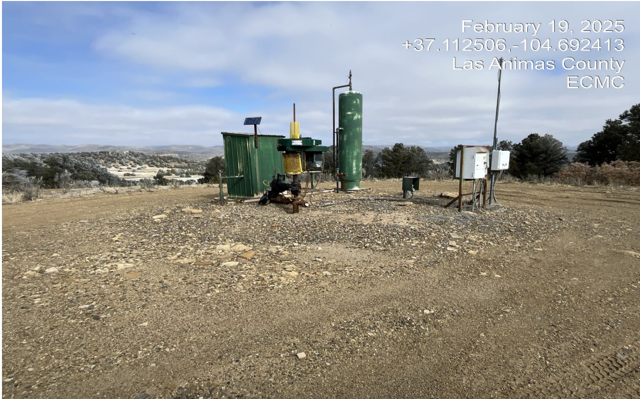
Photo 3. Facing toward the wellsite equipment.
