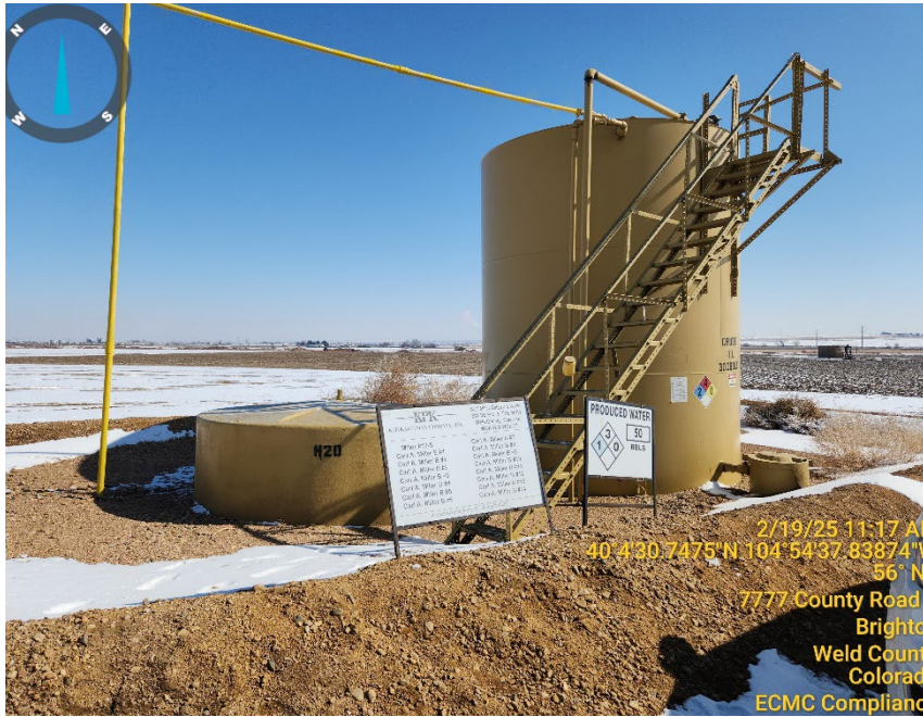
Photo 5: Centralized tank battery
