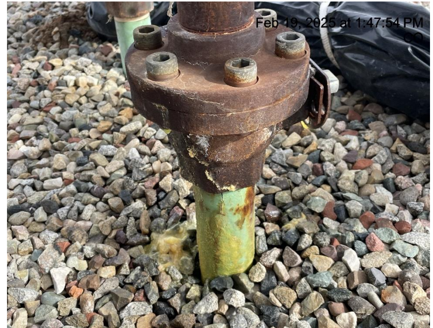
Photo # 7405 Mechanical condition – possible valve leak
