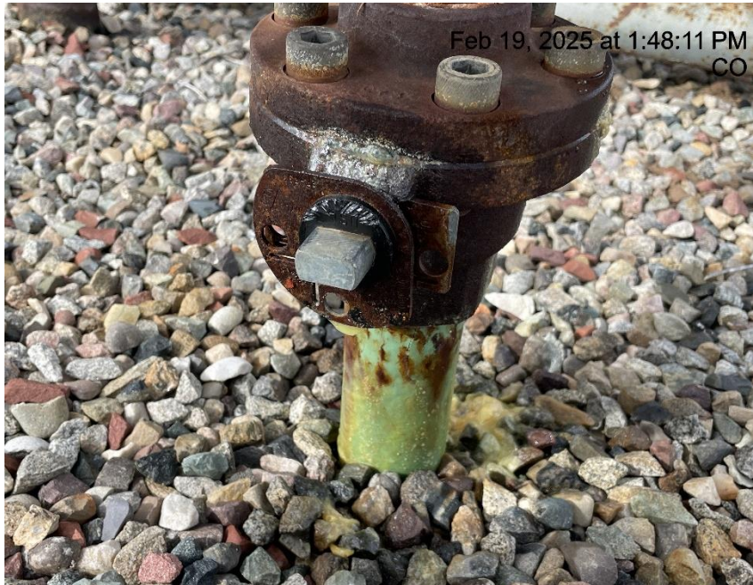
Photo # 7404 Mechanical condition – possible valve leak
