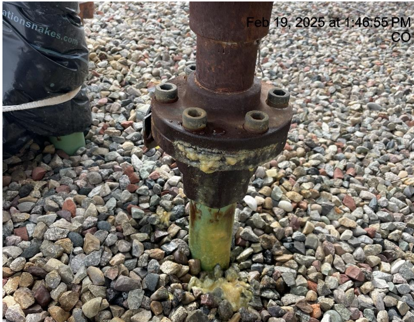
Photo # 7406 Mechanical condition – possible valve leak
