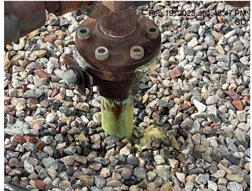
Photo # 7403 Mechanical condition – possible valve leak
