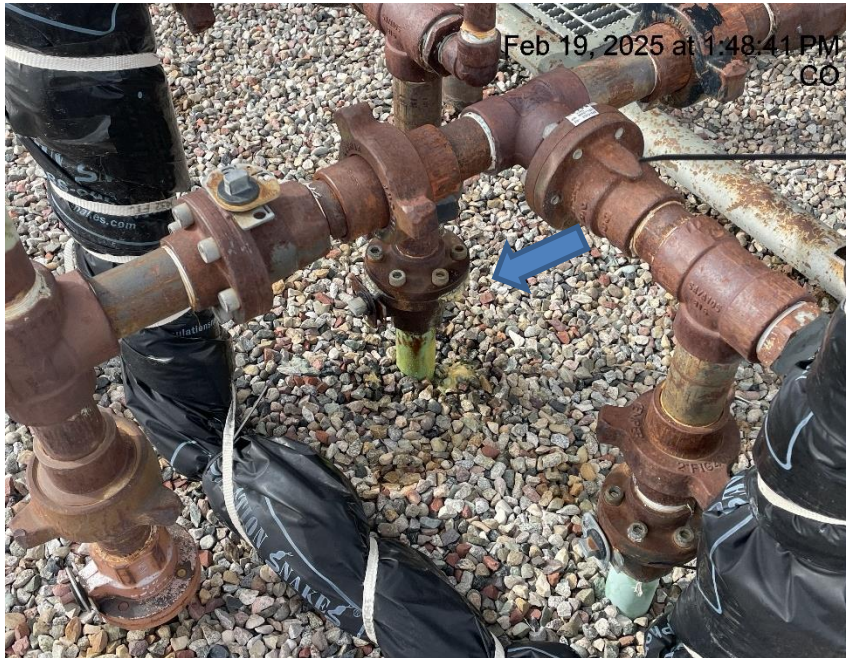
Photo # 7402 Mechanical condition – possible valve leak
