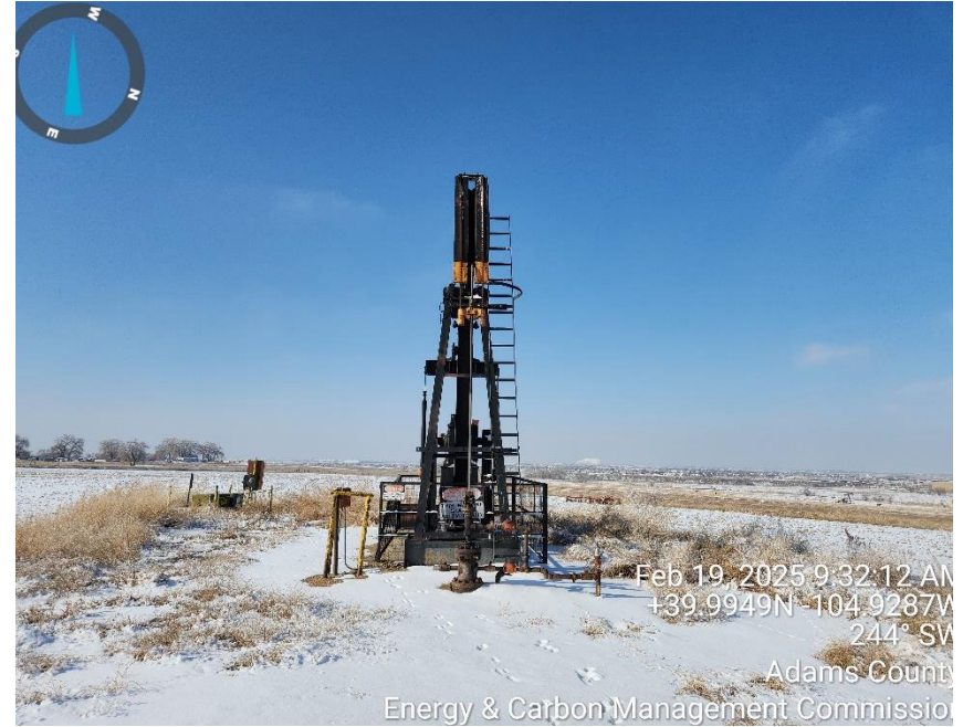
Photo 2 well head and equipment
