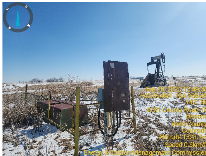
Photo 4 Electric panel & meter box are shut off.
