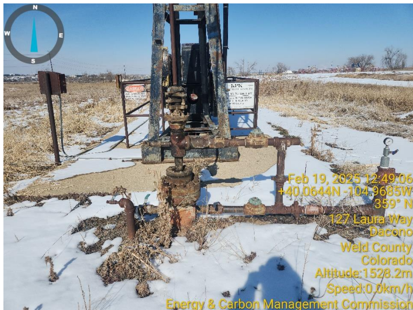
Photo 3 Wellhead valves are closed.
