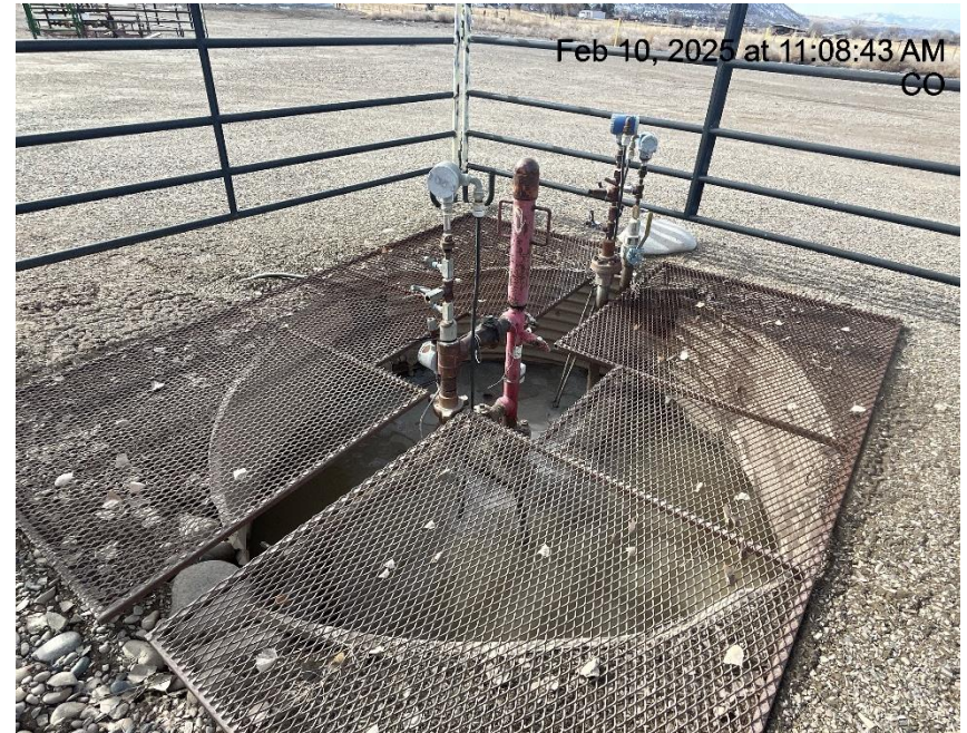
Photo # 4461 Cellar lacks wildlife egress
