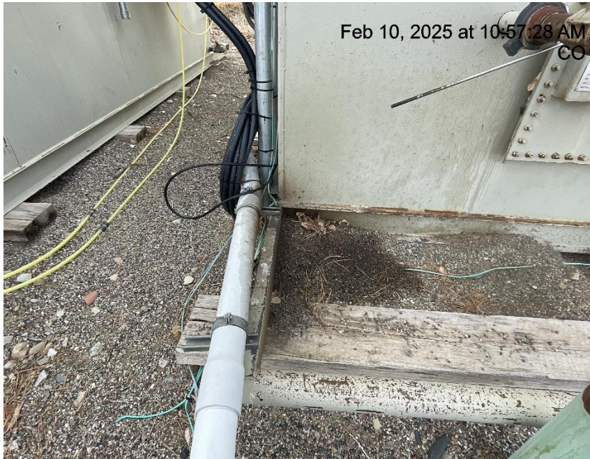
Photo # 4458 Staining near separator
