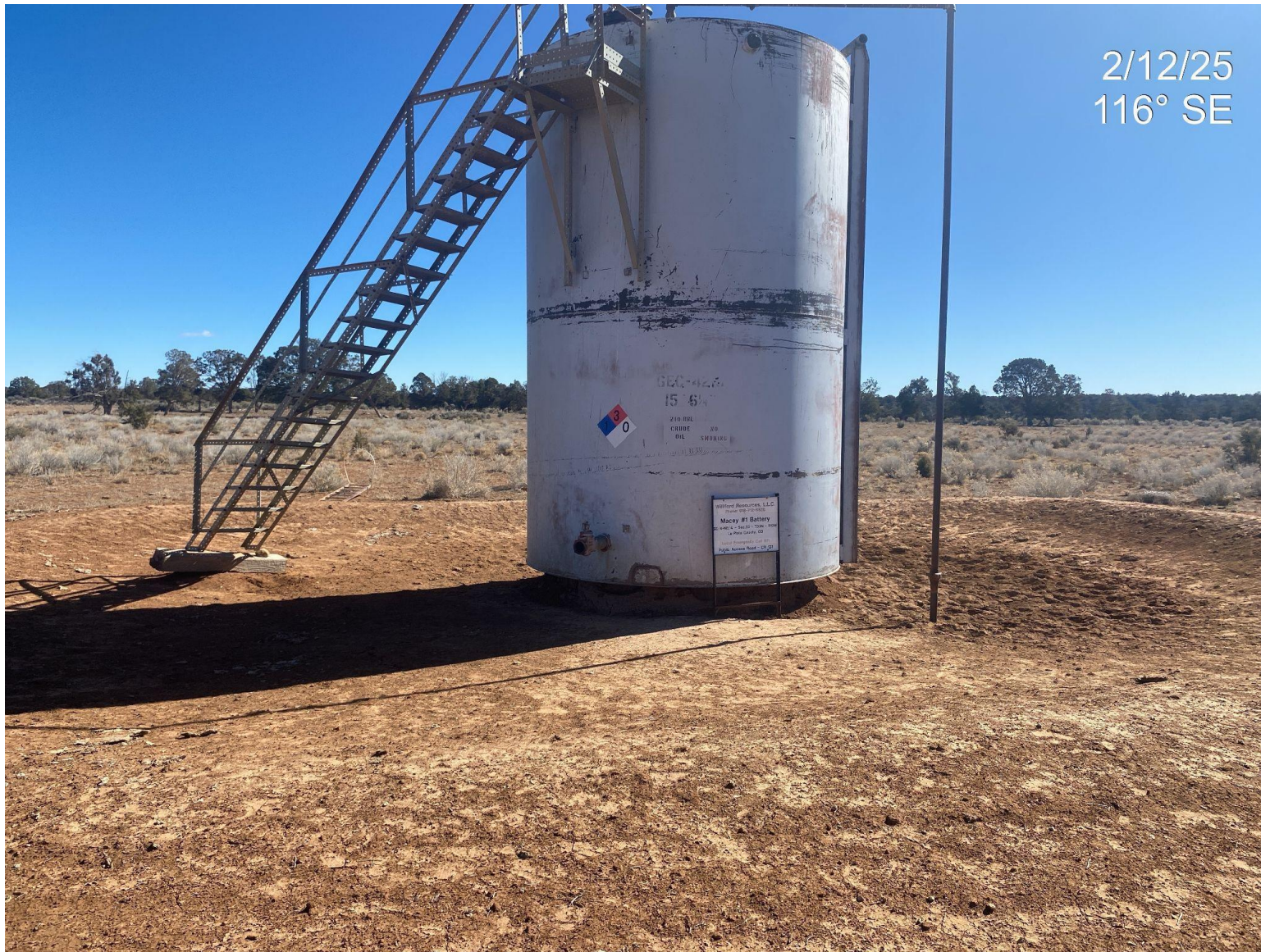
Photo 2. View of tank battery.
