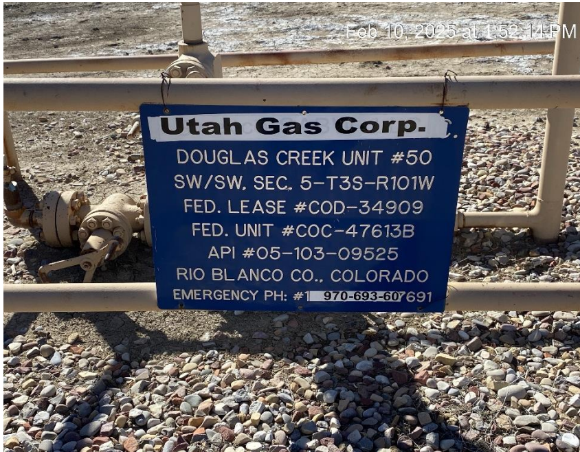
Emergency number needs replaced
