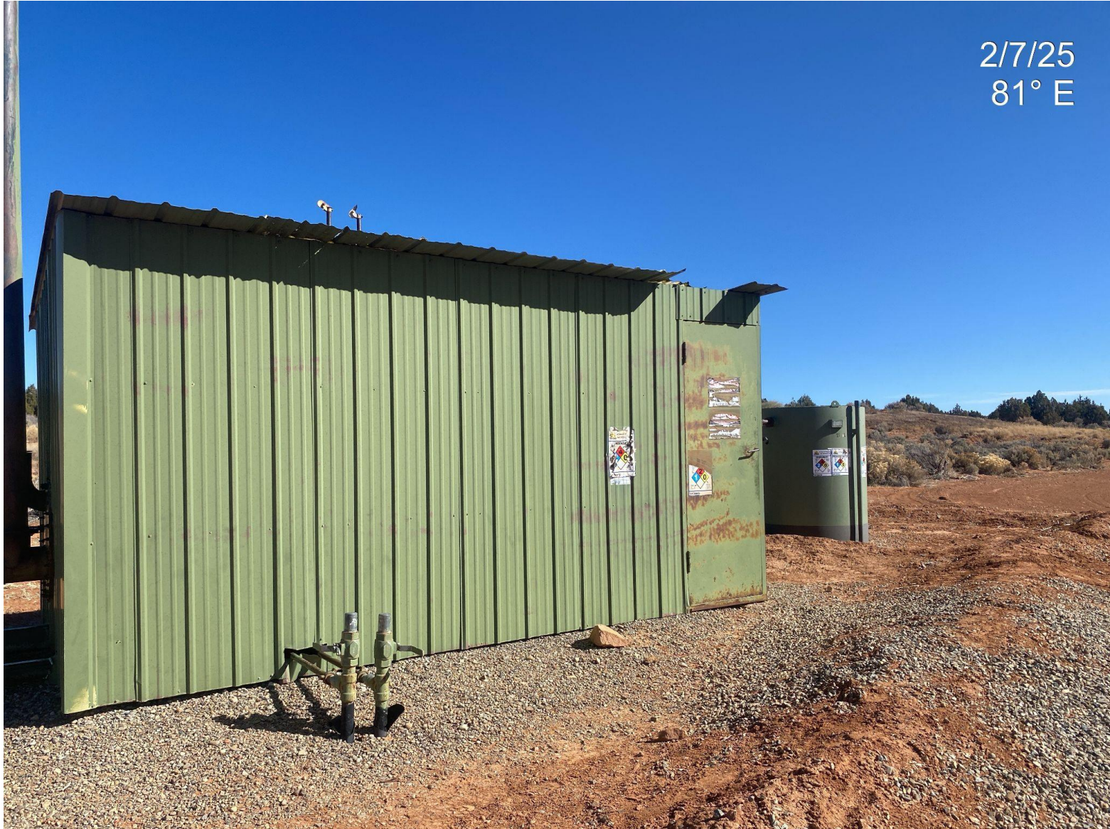
Photo 3. Labels at shed/separator equipment are starting to deteriorate, future maintenance advised.
