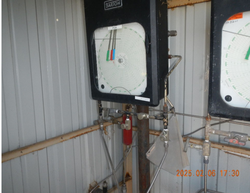
5. Gas meter inside meter shed.
