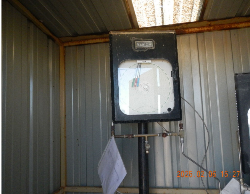
5. Gas meter inside meter shed.
