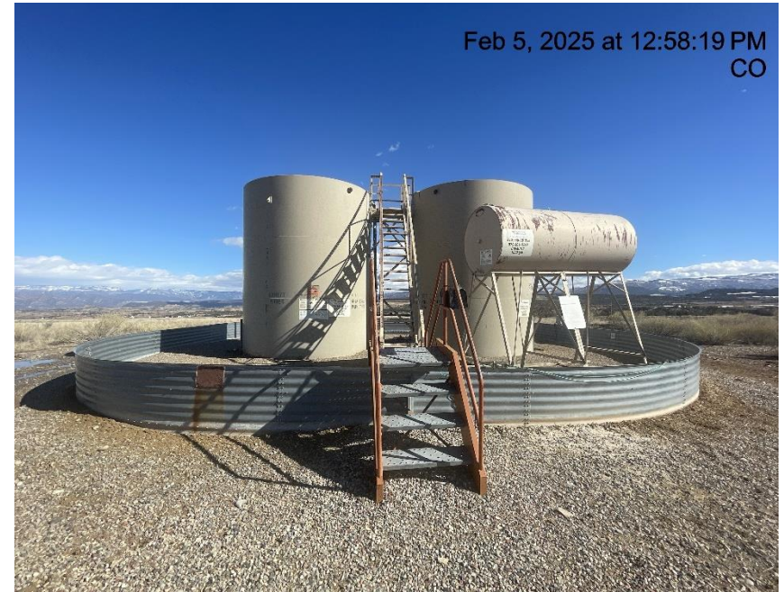
Photo # 3684 Battery lacks required signage/not in compliance with CECMC rules
