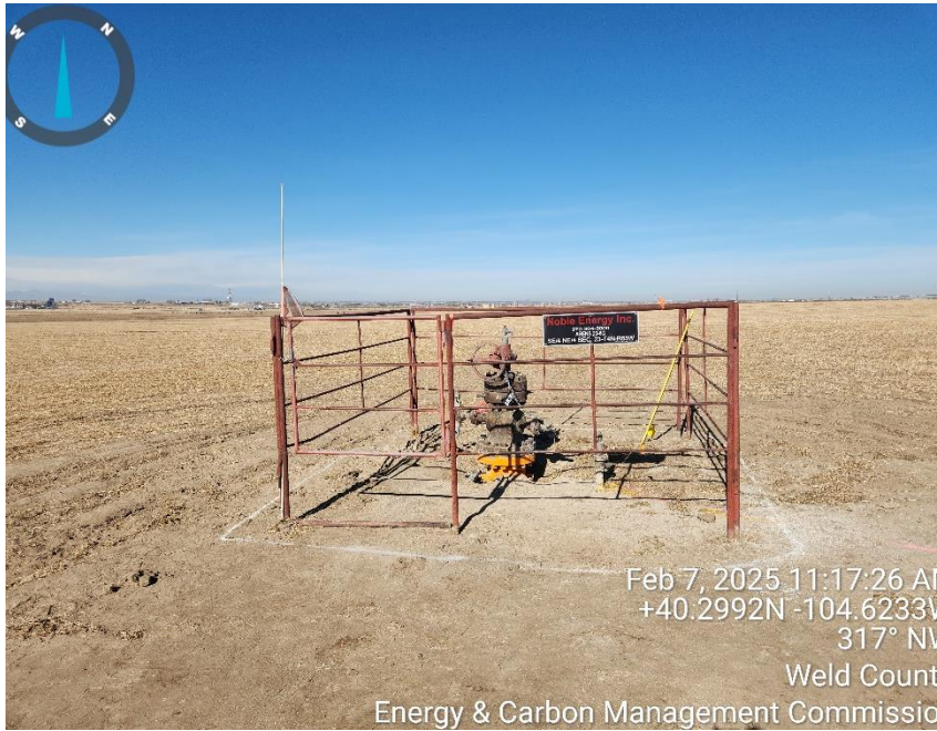
Photo 1 well head and equipment
