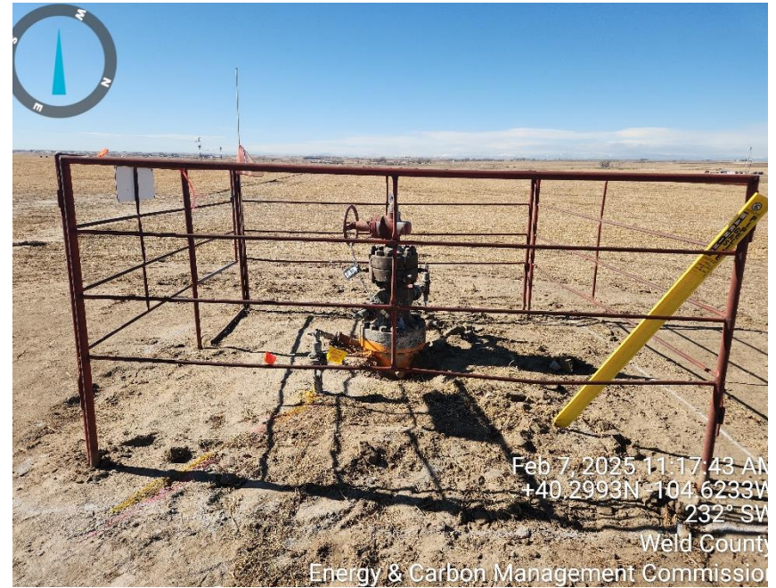
Photo 2 well head and equipment
