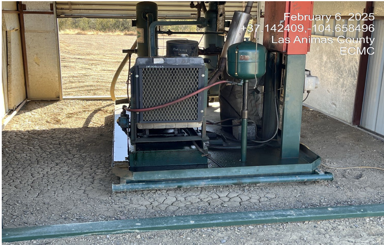
Photo 4. There is some oily fluid in the engine skid that will need to be cleaned up..
