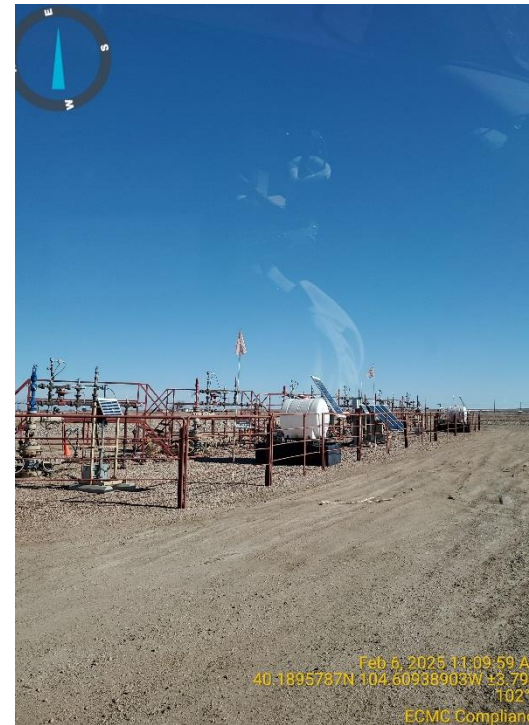
Wellheads and Corrosion Inhibitor Chemicals
