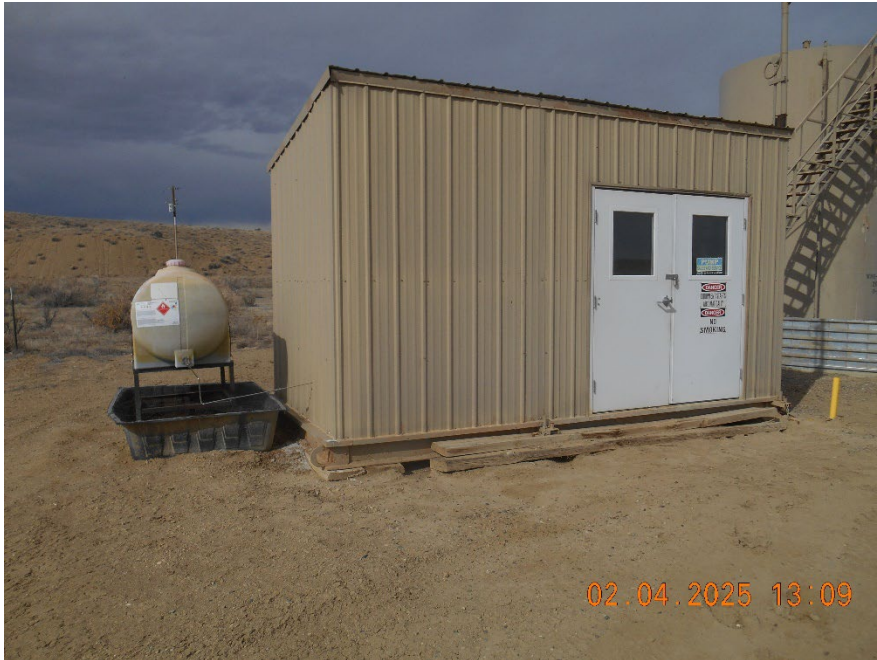
Pump housing. Secondary containment of chemicals
