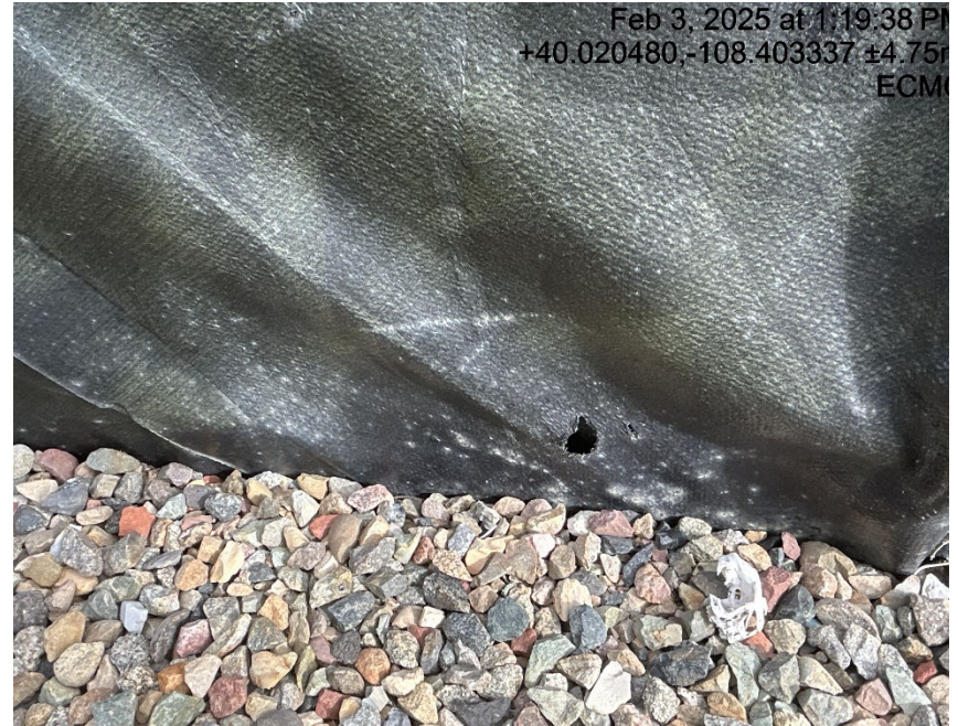
Hole in liner
