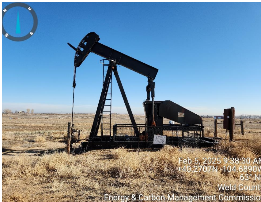
Photo 1 well head and equipment
