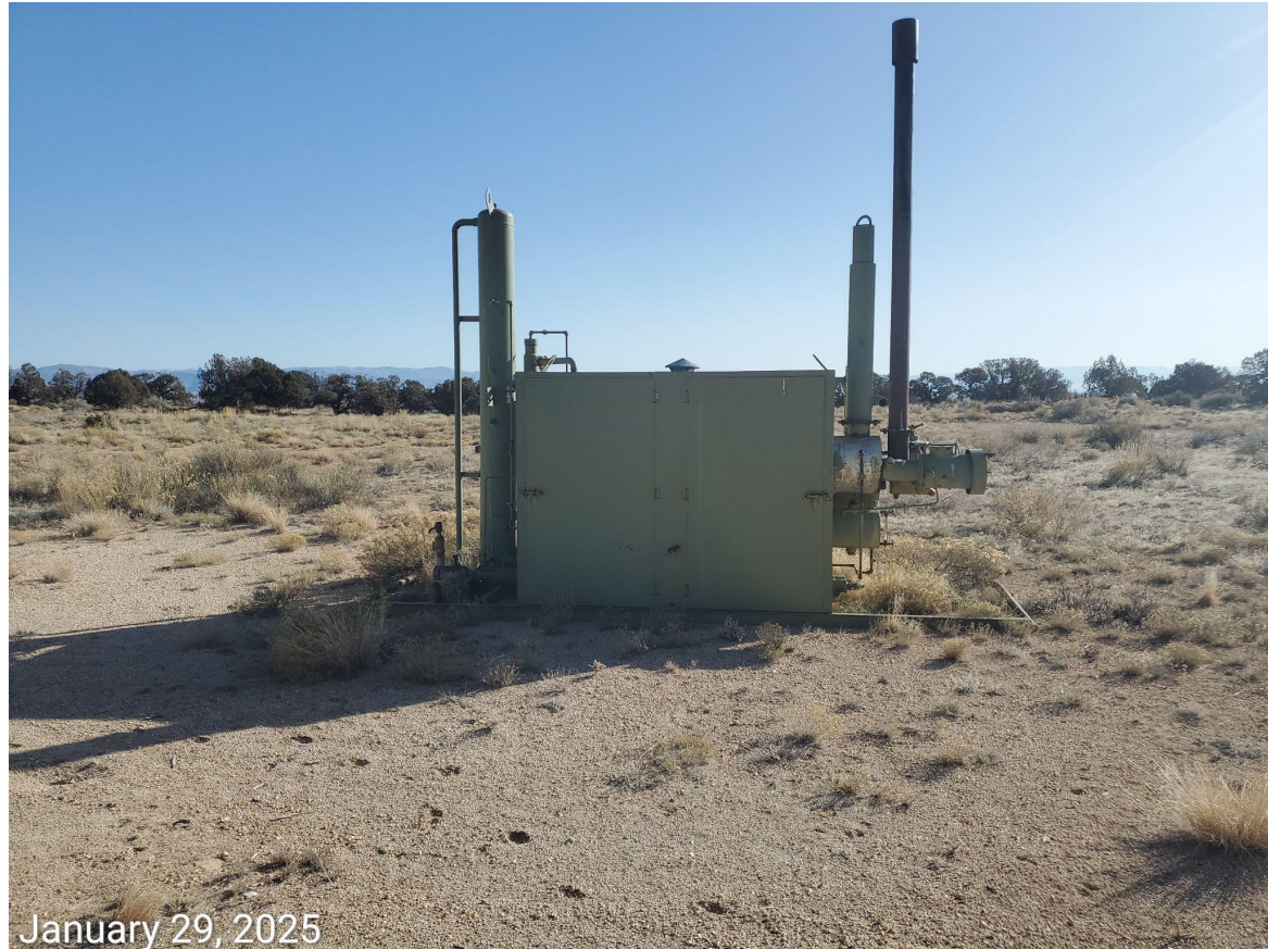
Photo 3: Separator equipment remaining on the west end of the Location.
