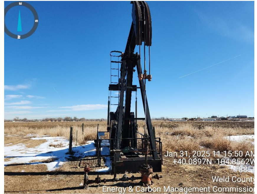
Photo 2 well head and equipment
