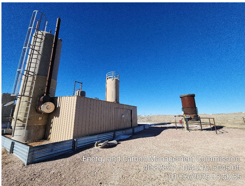
Photo 3 – Heater Treaters and ECD
