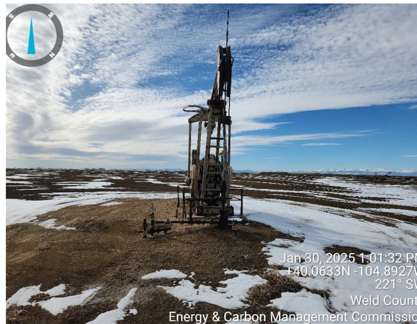
Photo 2 well head and equipment
