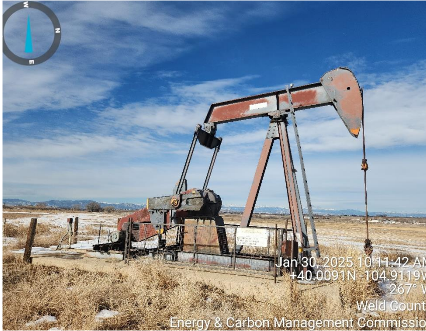
Photo 1 well head and equipment
