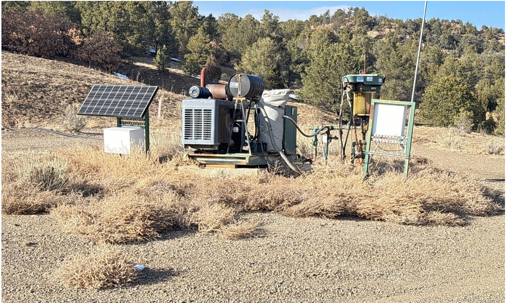
PHOTO 3: WEEDS NEED TO BE MAINTAINED IN ACCORDANCE WITH RULE 606.
