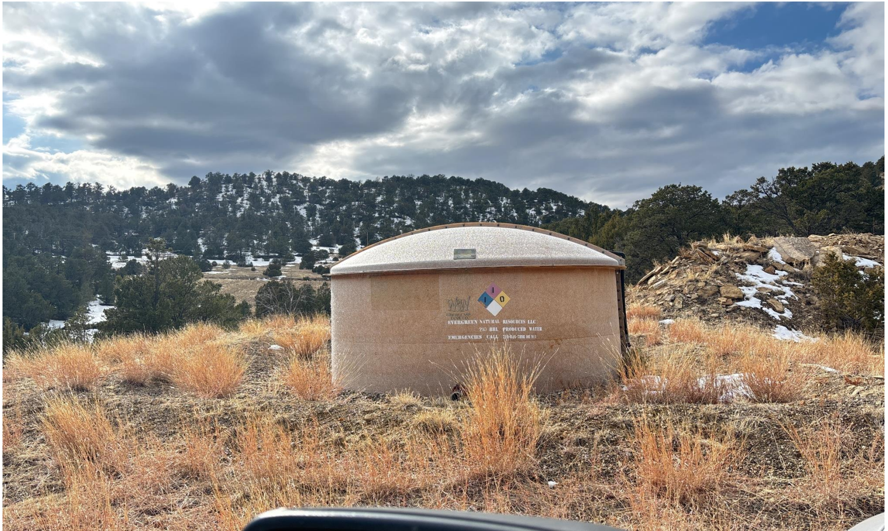
PHOTO 4: WEEDS ON AND INSIDE TANK BATTERY SECONDARY CONTAINMENT BERMS NEED TO BE REMOVED.
