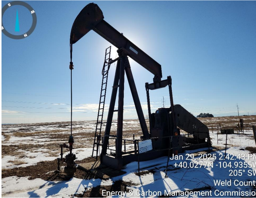
Photo 1 well head and equipment
