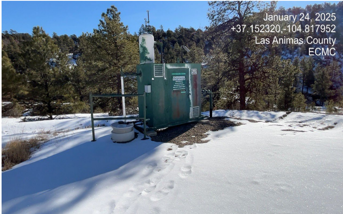
Photo 3. The well sign is posted on the meter shed.
