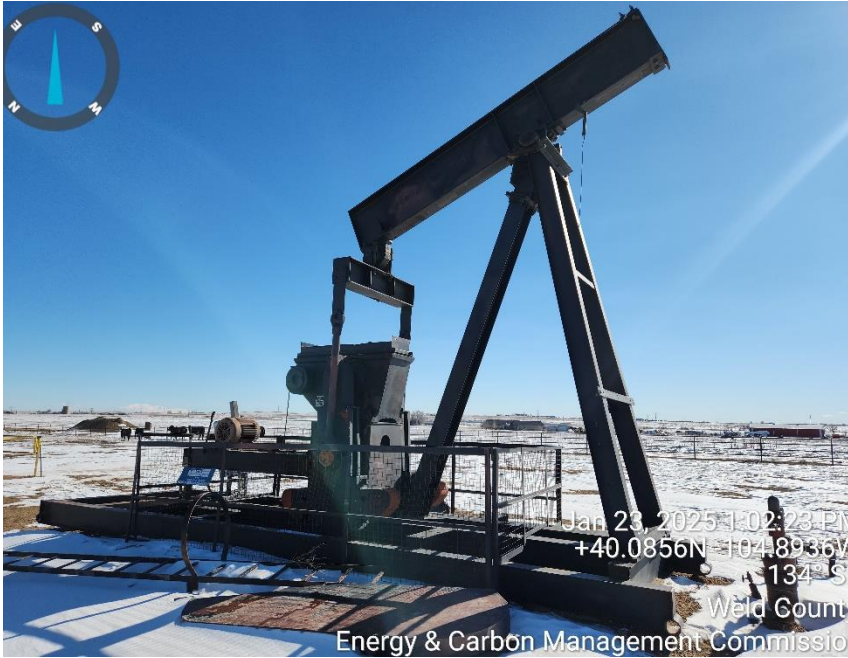
Photo 1 well head and equipment
