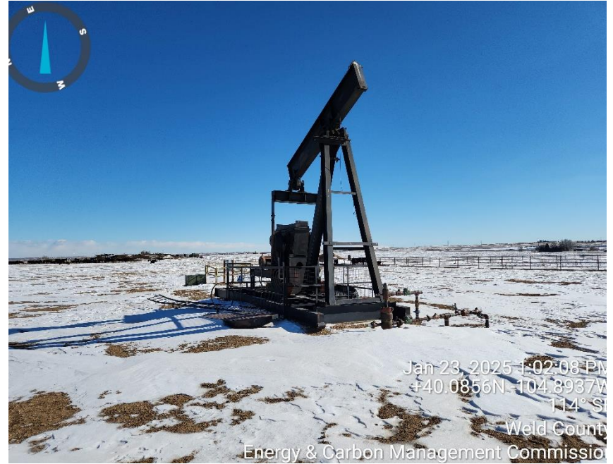
Photo 2 well head and equipment
