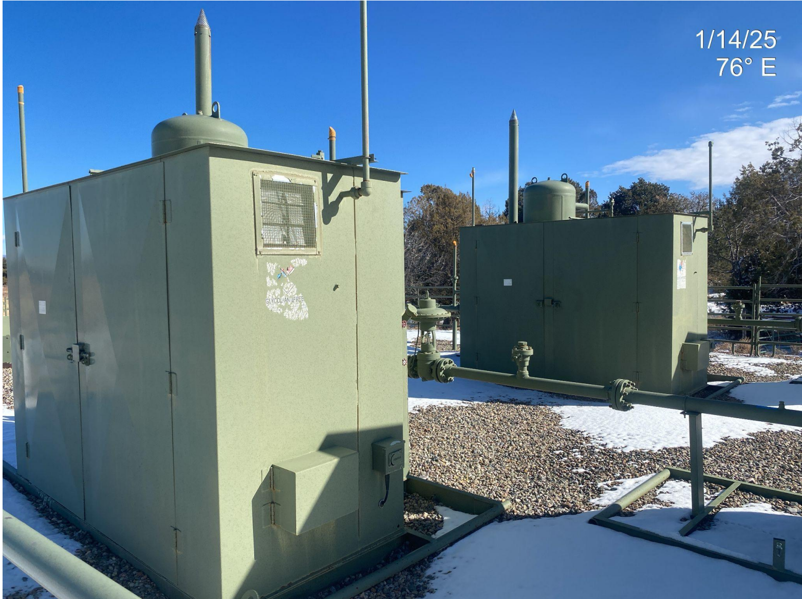
Photo 4. Label at separator has deteriorated and is no longer legible.
