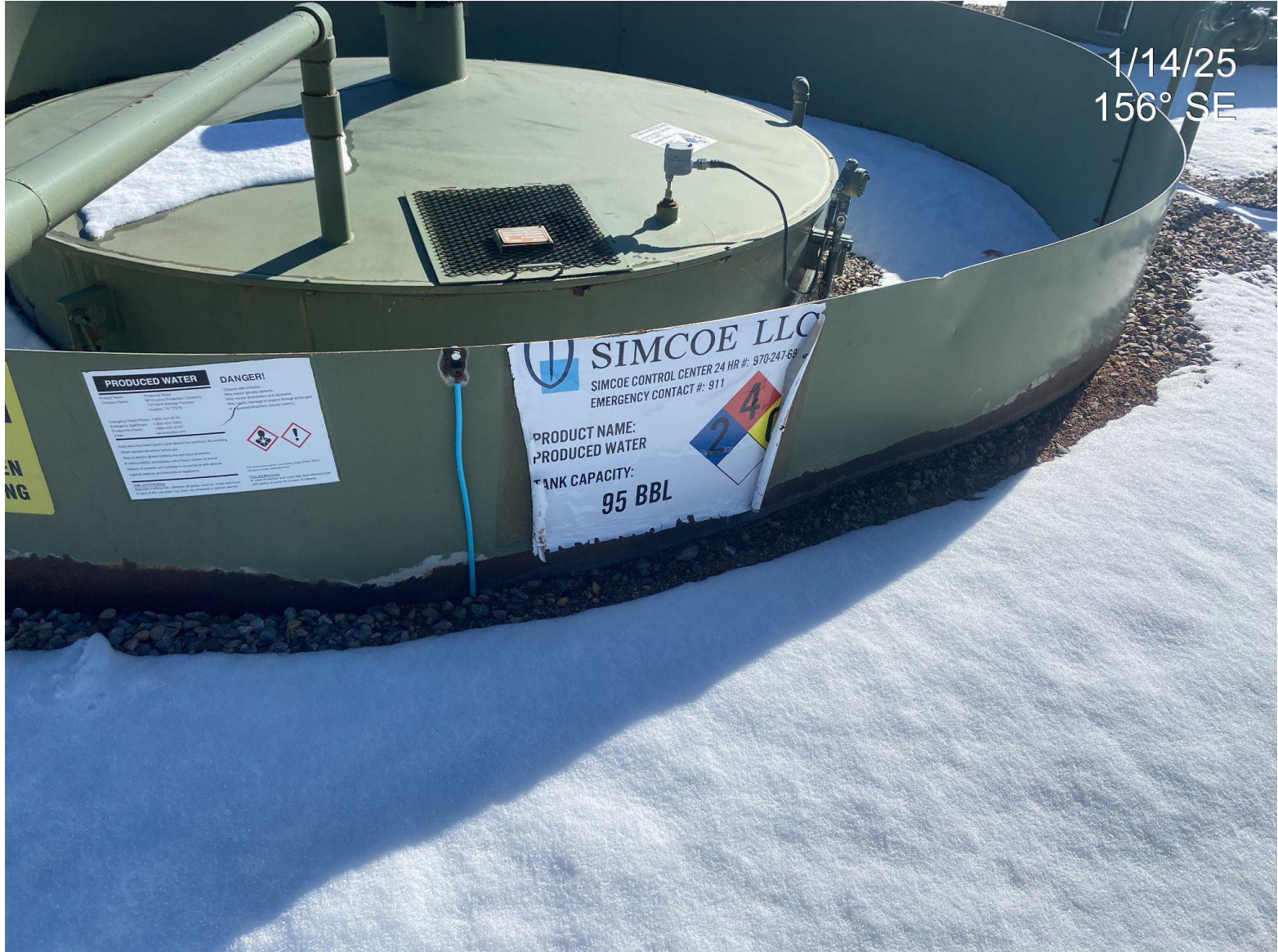
Photo 3. Produced water tank label is peeling, future maintenance is advised.
