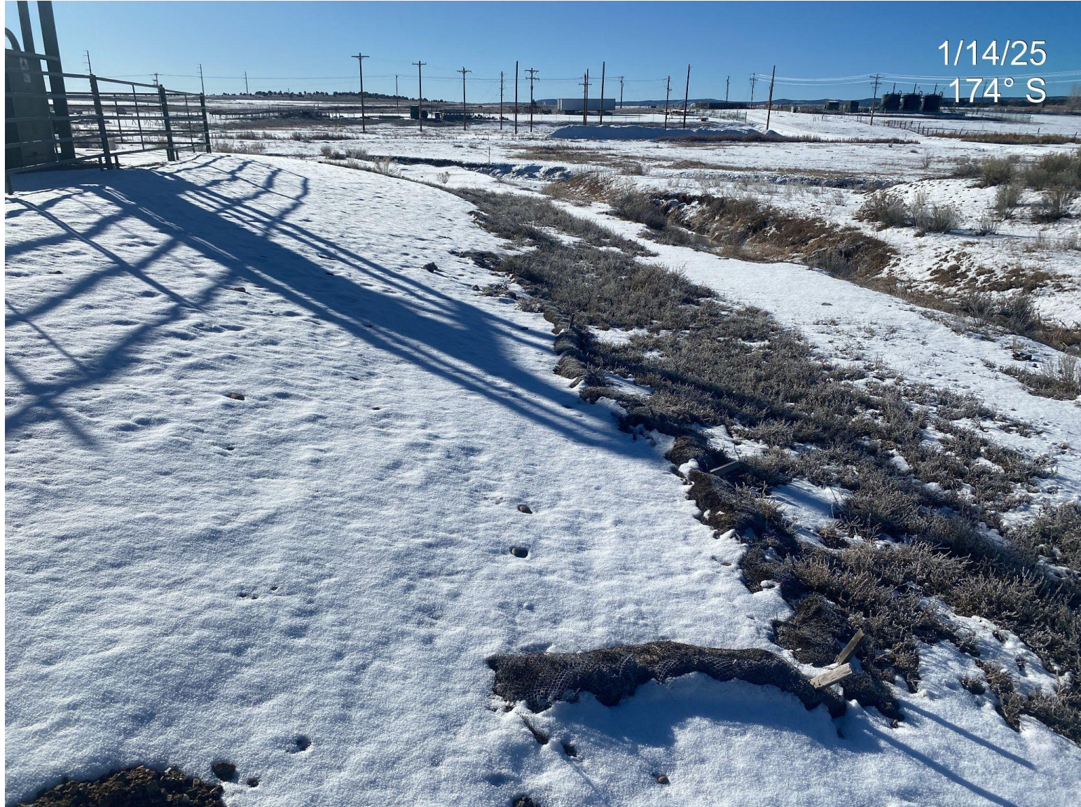
Photo 2. Wattles on the western edge of the pad are disintegrating are not longer functioning.
