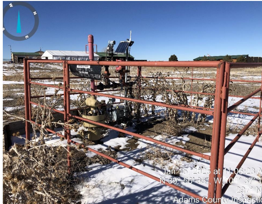
Photo #3 Well head
