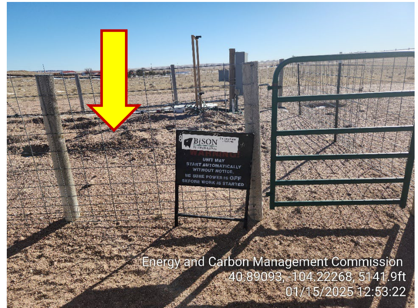
Photo 4 – Well Sign missing
