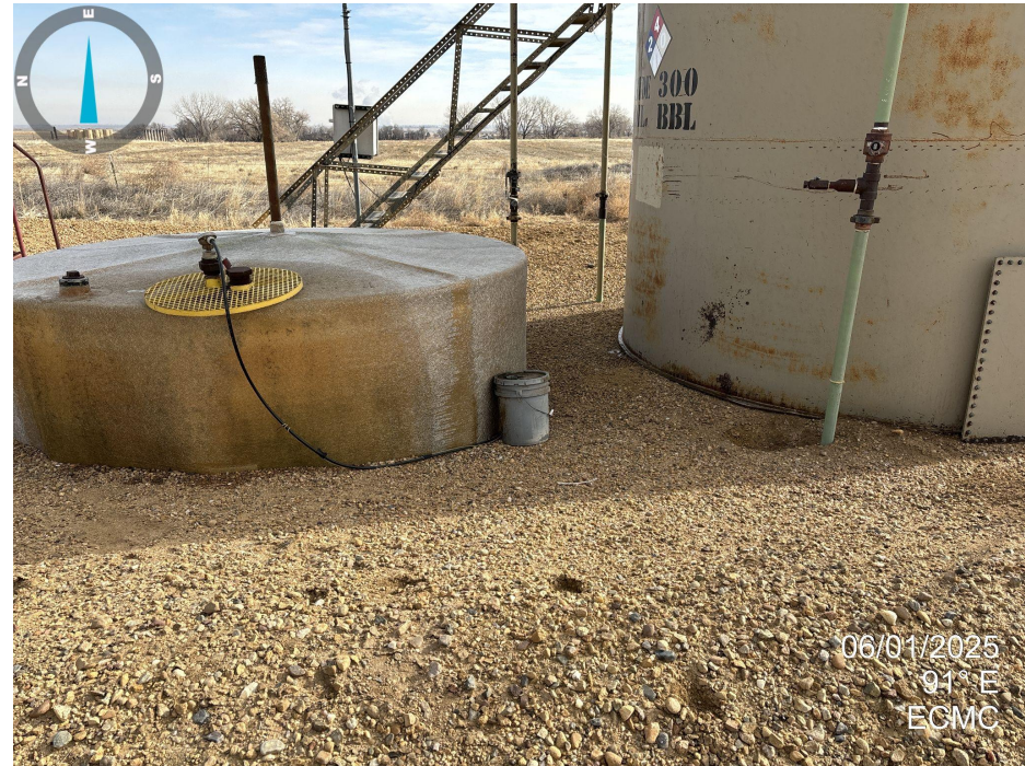
Photo 4. Open bucket containing oily waste near partially buried produced water tank.
