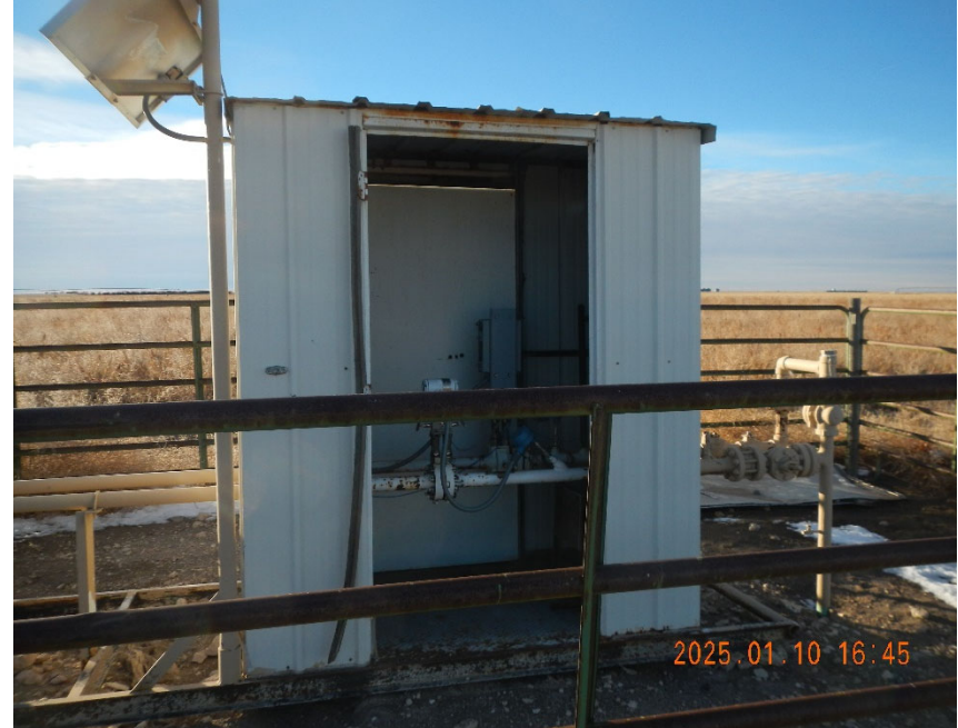
4. View of meter shed missing door. Door is on ground inside fencing.
