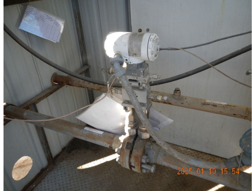
6. Gas meter inside meter shed.
