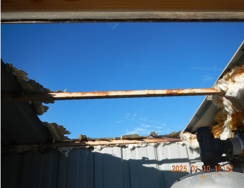
5. Roof damage on separator shed.
