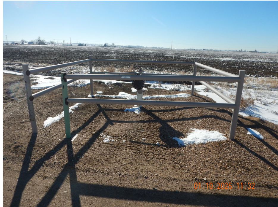
Photo 2. Photo illustrates aboveground midstream equipment remains and appears to be active.
