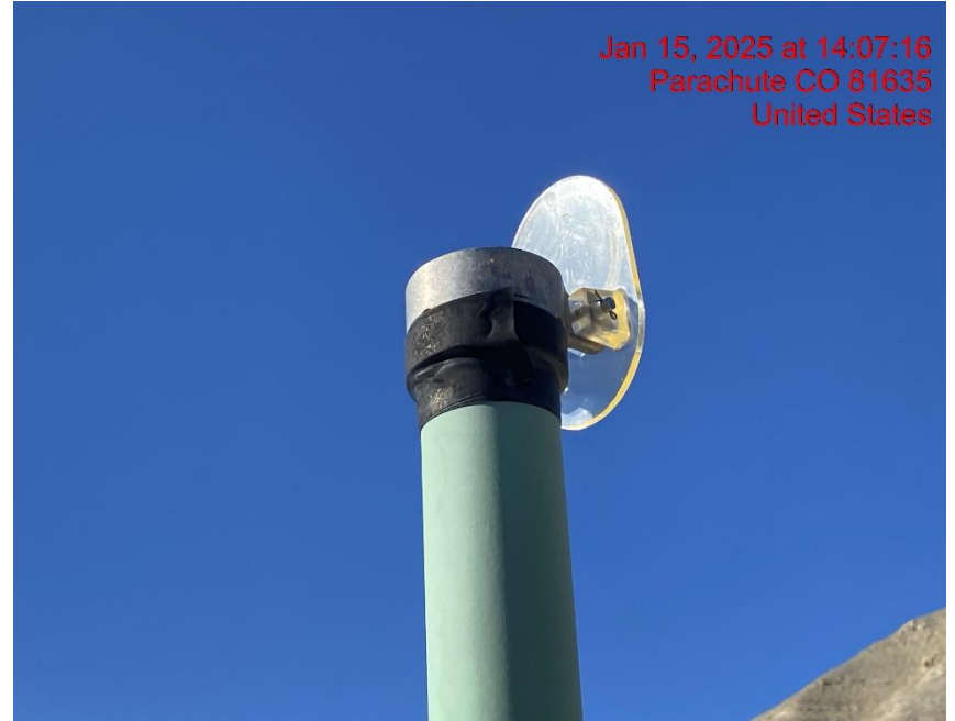
Vent Cover Stuck Open – Photo #06010
