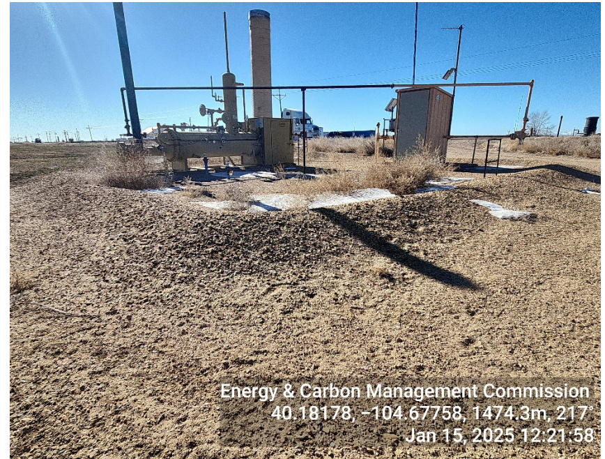
Photo 8: Dead, overgrown vegetation/debris. Not maintained earth berm
