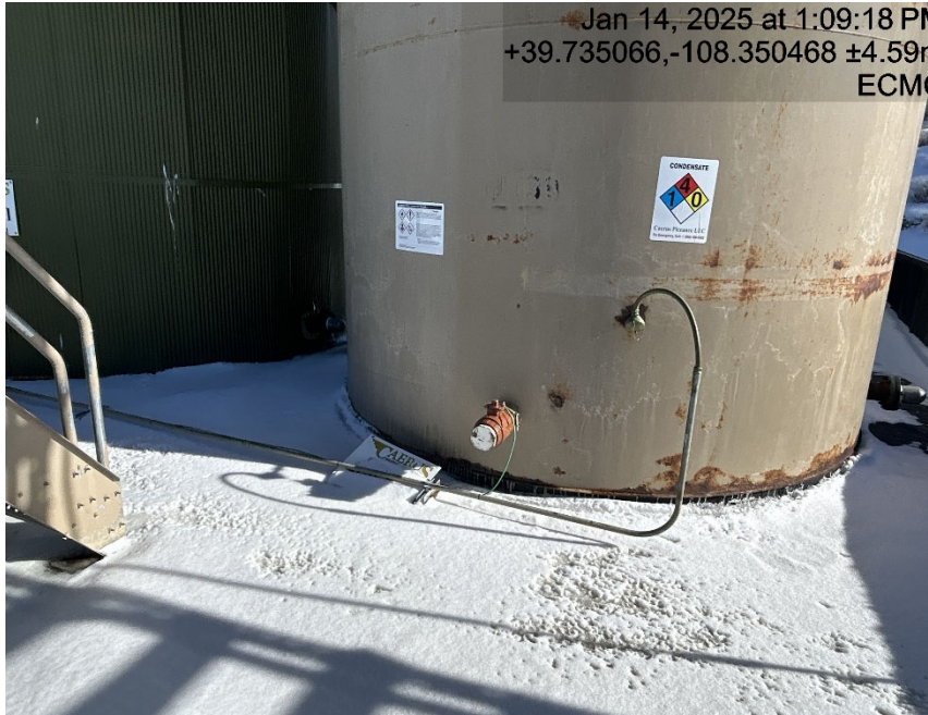
Tank signage fallen off
