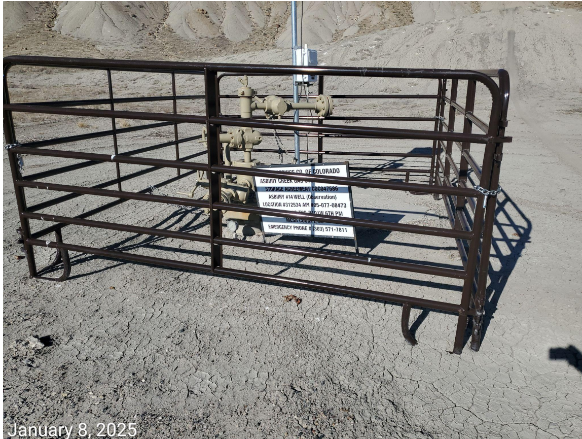
Photo 2: Well on Location.
