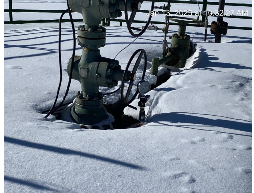
Gap and open space in cellar cover
