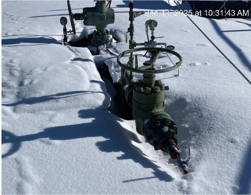
Gap and open space in cellar cover
