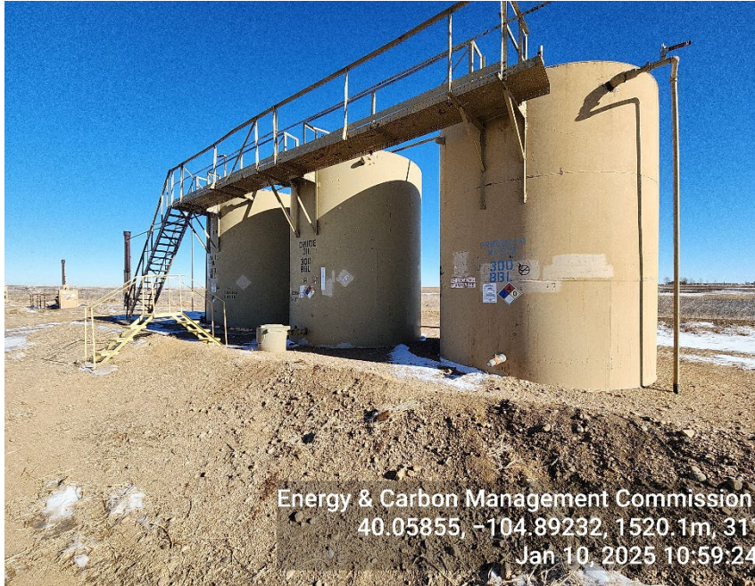
Photo 3: Centralized tank battery
