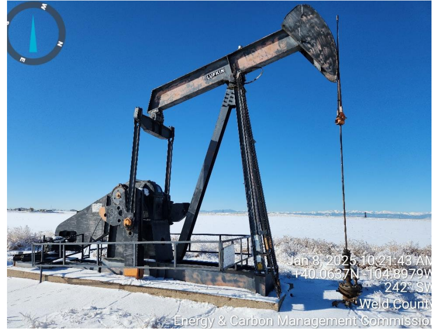
Photo 2 well head and equipment
