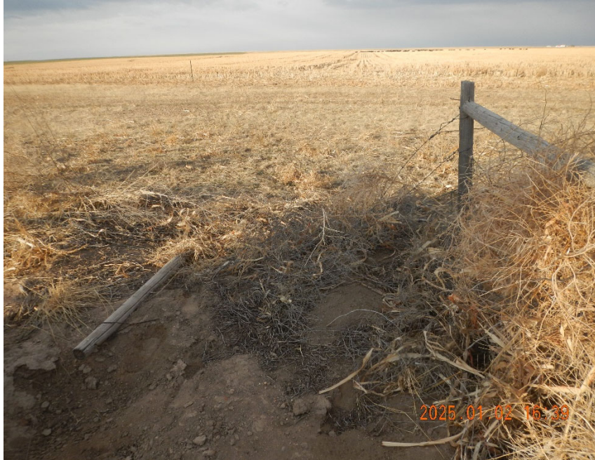
7. View of portion of fencing down at remote gathering location. Post has rotted off.
