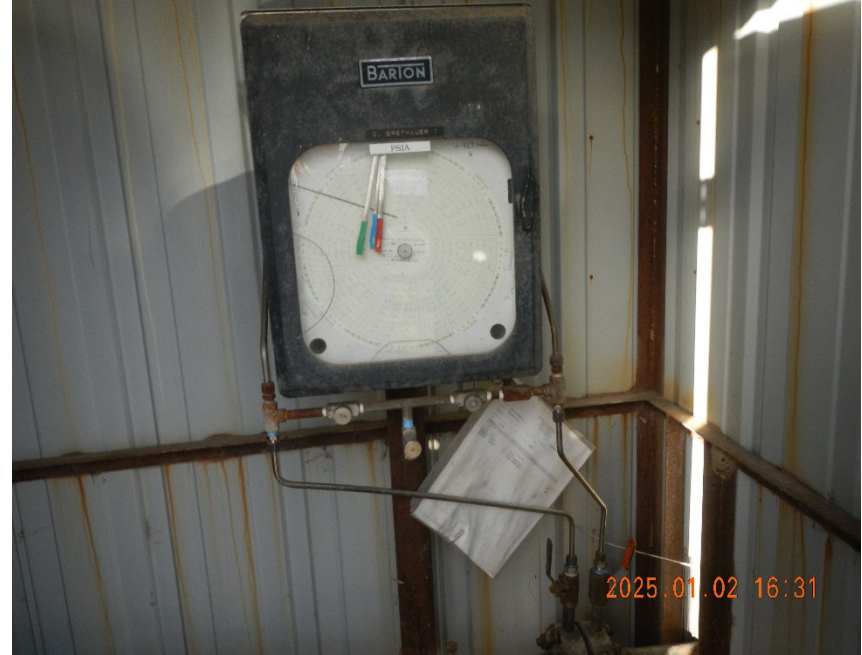
6. Gas meter inside shed.
