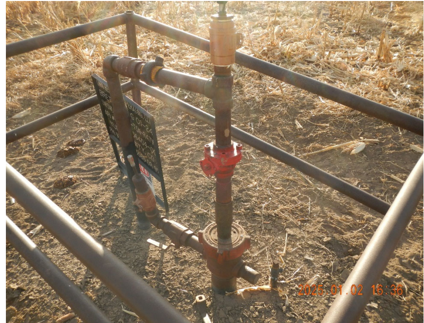
2. View of wellhead.
